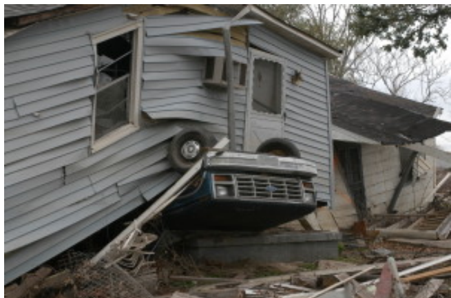
Katrina Damage Photo: Russ Curtis
